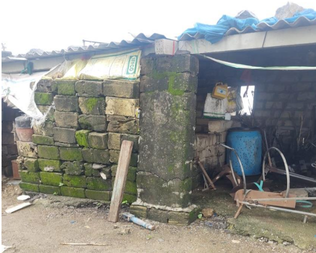
Fig. 1: House of deceased: typically, kaccha type temporary settlement with cracks and crevices
